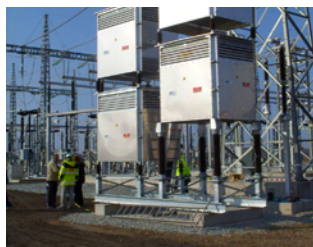
East Link, HVDC connection between Estonia and Finland.
