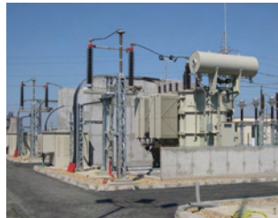
Neutral Earthing resistor, Romania.
